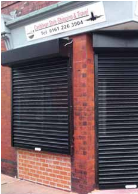
Image of bad grill shutter installations
